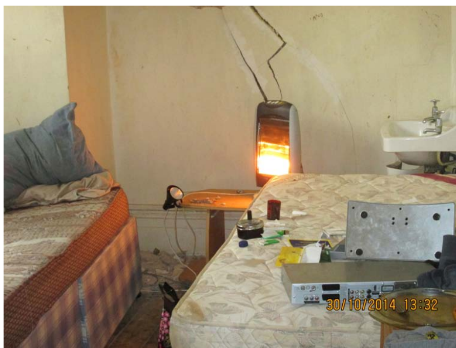
FIGURE 9: Rented property discovered through LB Lewisham's rogue landlords taskforce work
